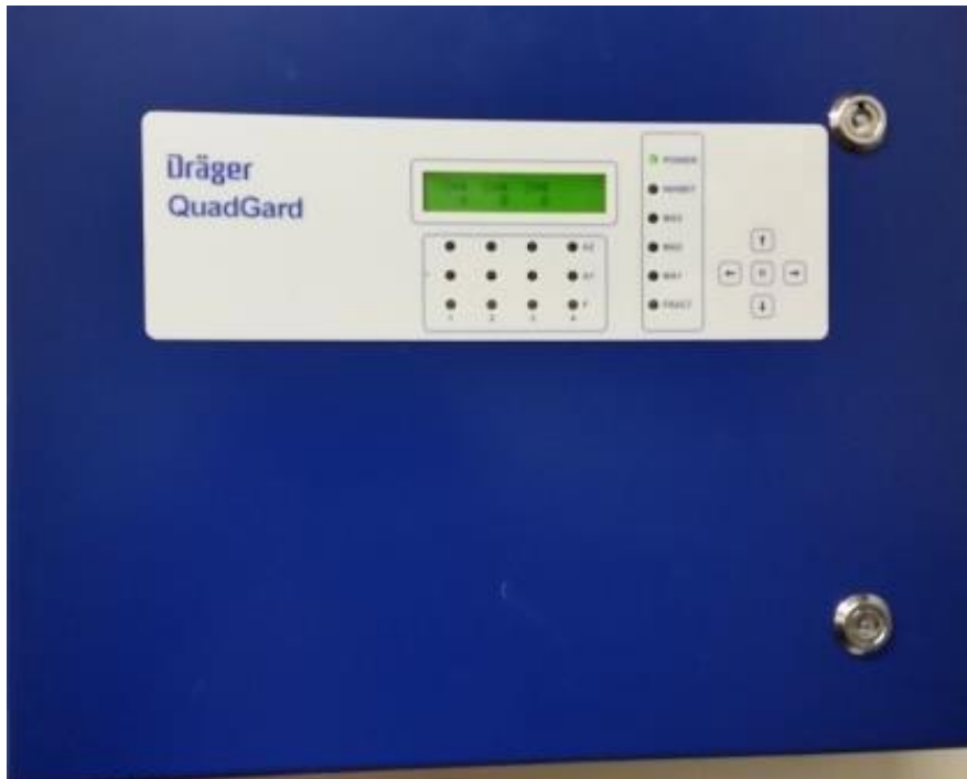
Figure 5.7 – GDGP-1 Control Panel (located in room B073B)
