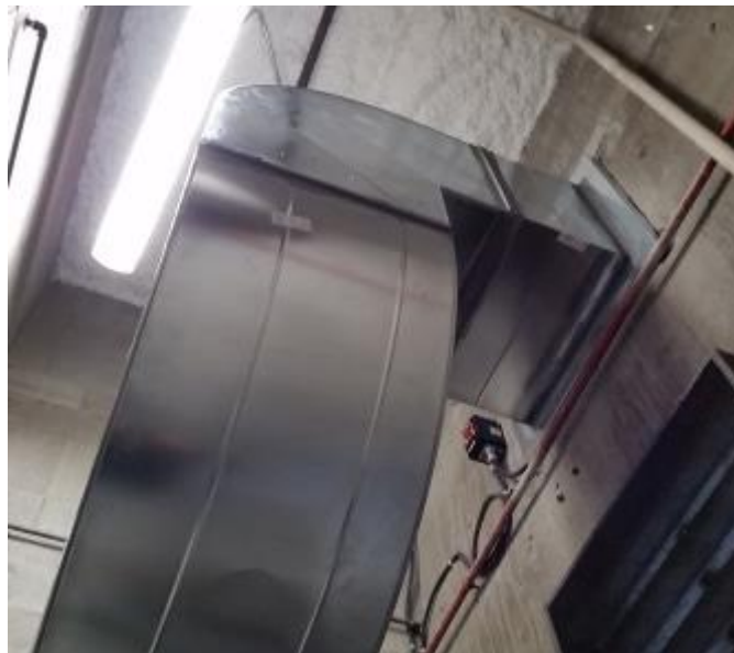
Figure 5.5 – Emergency Ventilation Ducting
