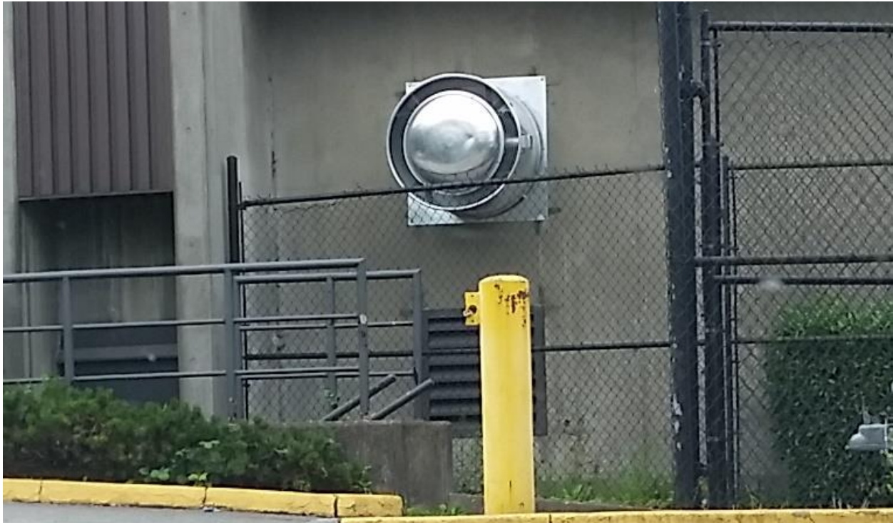
Figure 5.3 – Wall-mount Emergency Exhaust Fan (Room B080)
