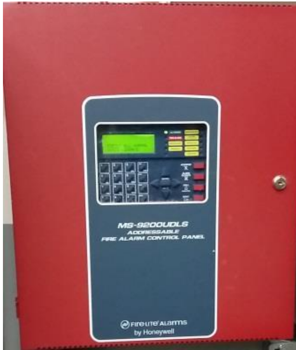
Figure 5.6 – FACP-1 Control Panel (located in Room B073B)
