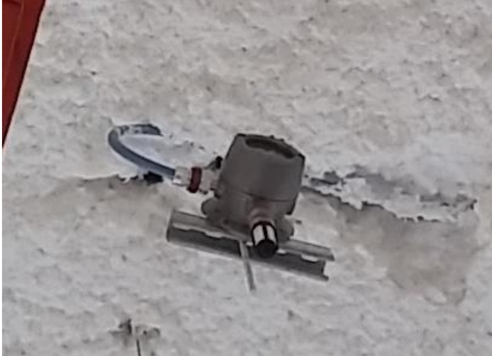
Figure 5.4 – Gas Sensor Ceiling Mounted
